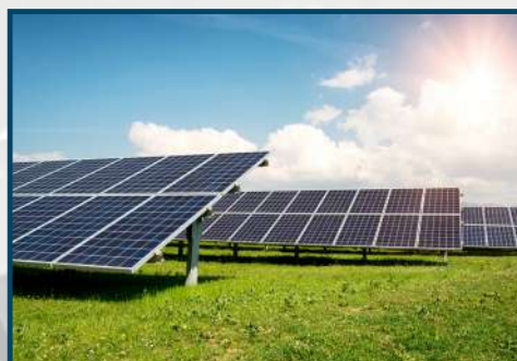
Pannelli solari / Solar panels
